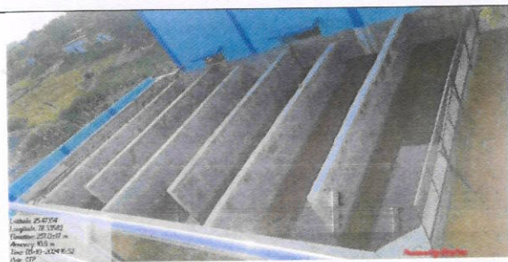
Pic.7: Chlorination Tank
