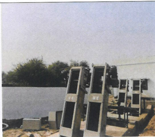
Pic.4: SPS 1 at Naya Gaon Nalla
