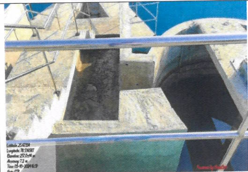
Pic.4: Grit Chamber
