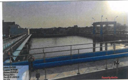
Pic.6: SBR Tank
