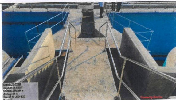
Pic.5: Parshall Flume
