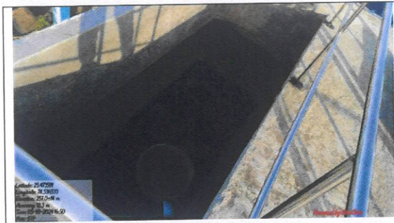
Pic.1: Inlet Chamber
